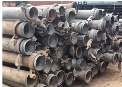
QD Piping, HDPE Piping, Hoses, & Fittings
