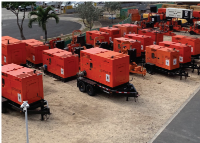
Dri-Prime Pumps for Sewer Bypassing & Dewatering
