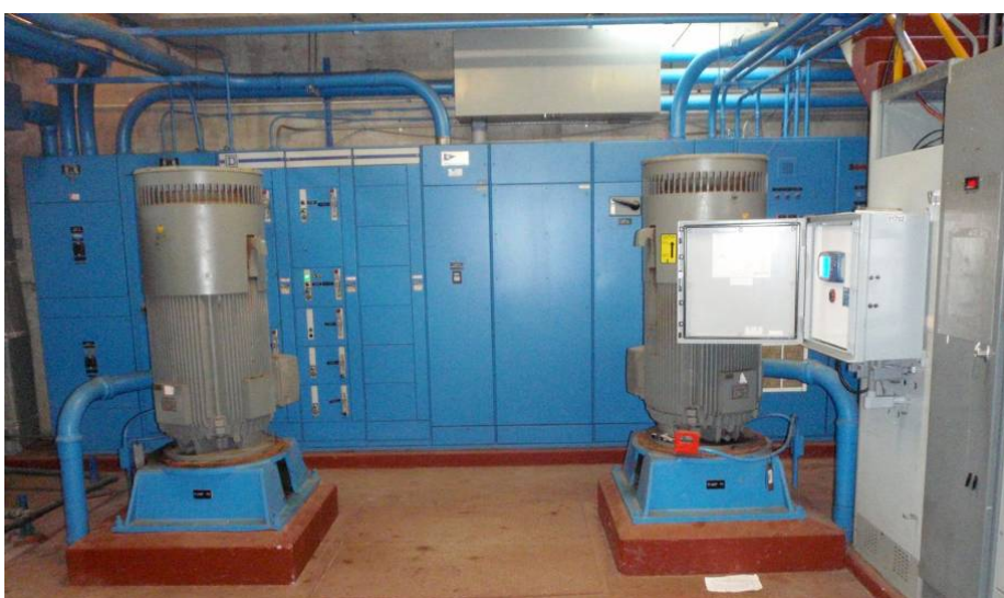
Lift Station at Aliamanu
