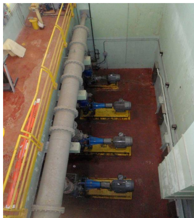
Lift Station at Fort Shafter
