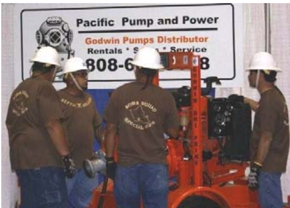
Maintenance Challenge: The teams prepare a Godwin Dri-Prime CD100M for service at a disabled lift Station.
