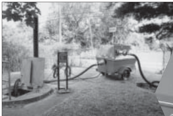
Municipal Pump Station Bypass
